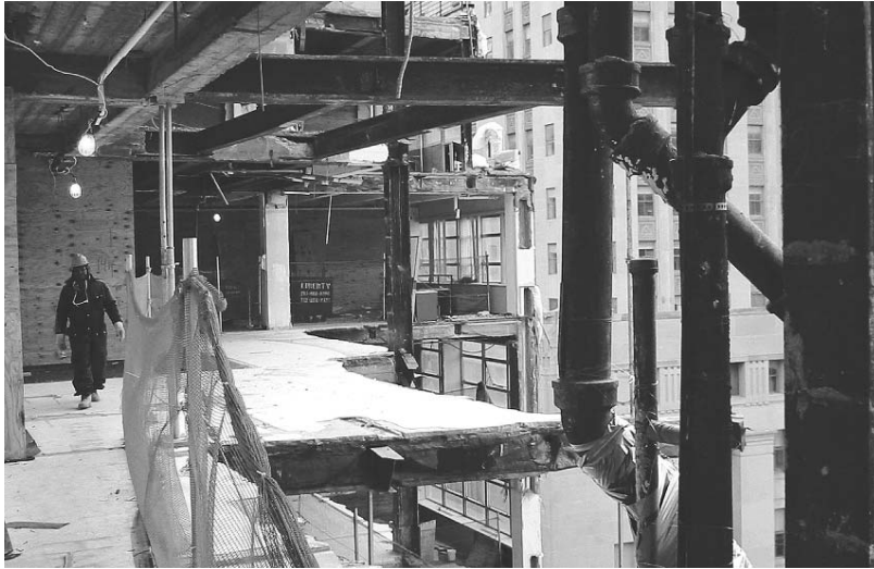
The view from inside Fiterman Hall, in January 2002, before the building was sealed off. Construction and safety workers demolished and removed loose parts of the building that might fall on pedestrians and crews at Ground Zero.
